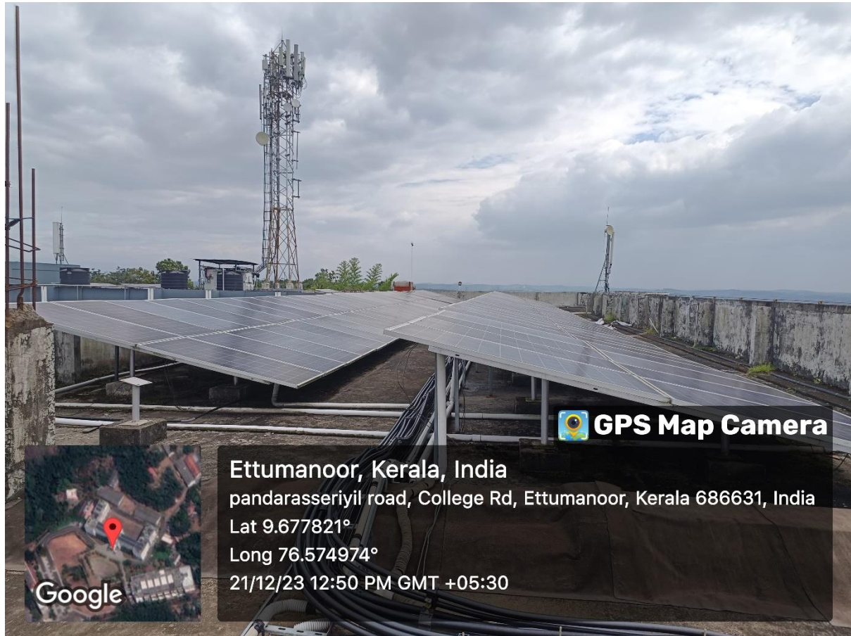
Fig 1, Solar Plant at the college
